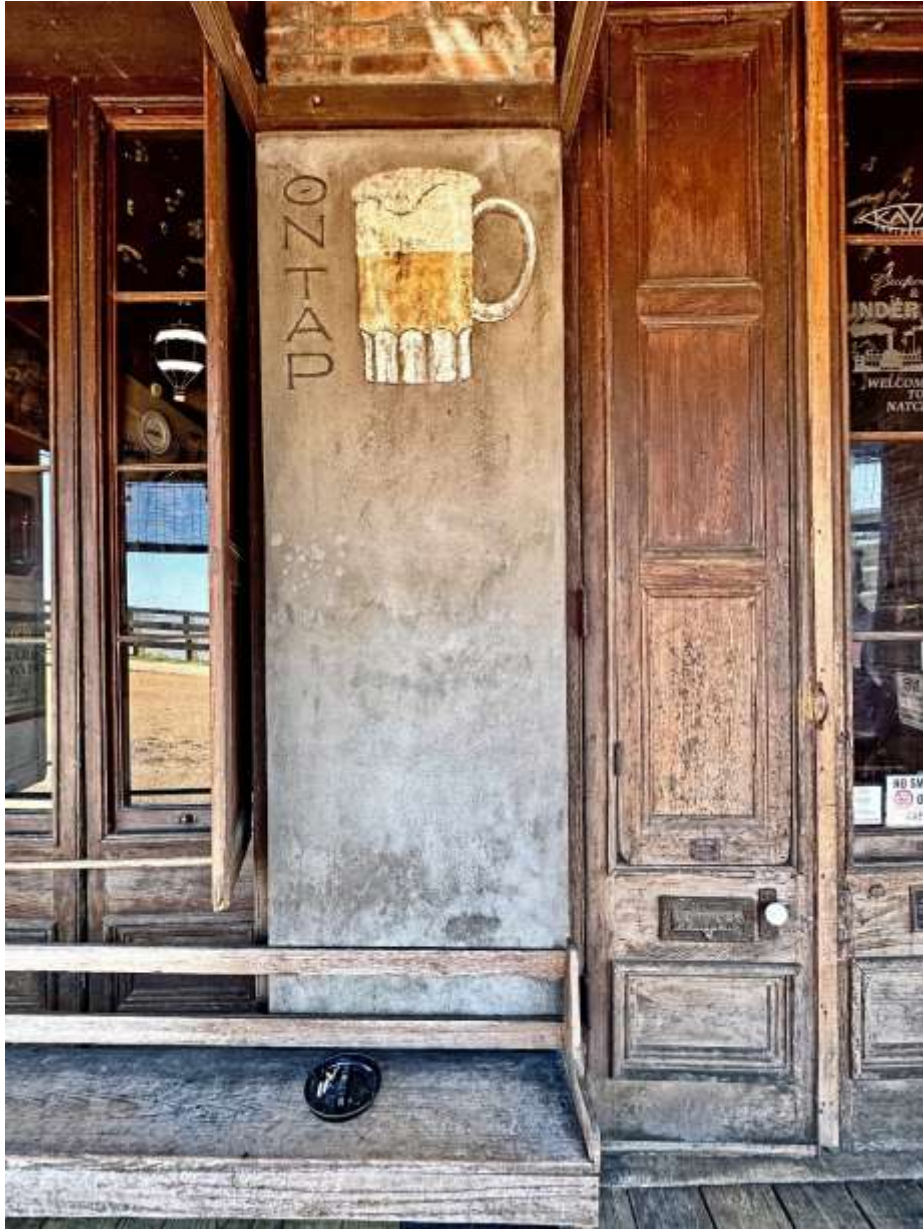
Exterior of Under the Hill Saloon —one of the oldest buildings in Natchez, MS built late 1700's or early 1800's. May 13
