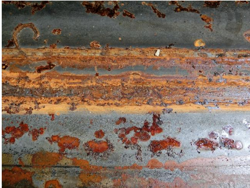
Rusted metal sheet
